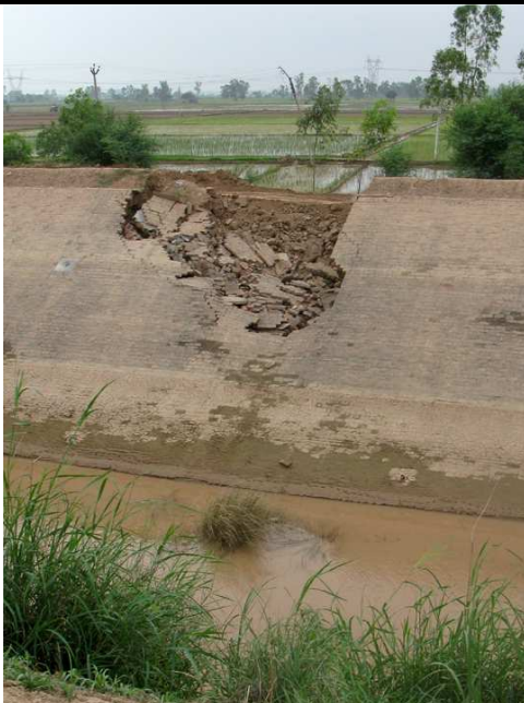
Another breach near Keorak on Hansi Butana Canal. Photograph taken on July 20, 2010.
