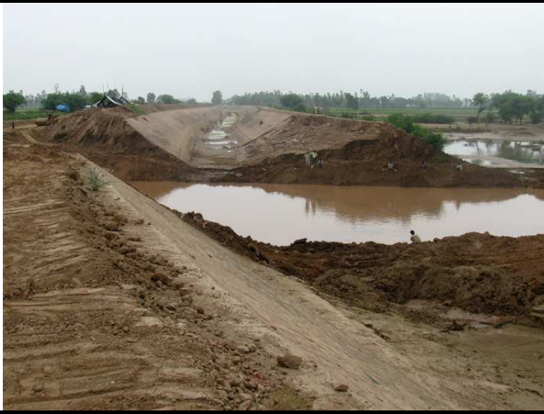
Breach on Hansi Butana Canal near Tatiana village, Kaithal District of Haryana on the midnight of July 7, 2010. Ghaggar water breached the Left bank of the canal and then breached the opposite bank also. Note the complete breakdown of the canal structure. River water enters from the left hand side and passes through right hand side. Photographed on July 21, 2010
