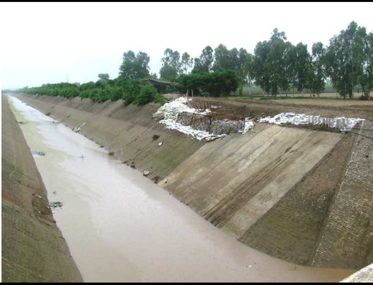
Breach on the right bank of the Hansi Butana Canal near Keorak village in Kaithal District of Haryana. Breach occurred on July 9, 2010. Temporary plugging is noticed. Photograph taken on July 20, 2010
